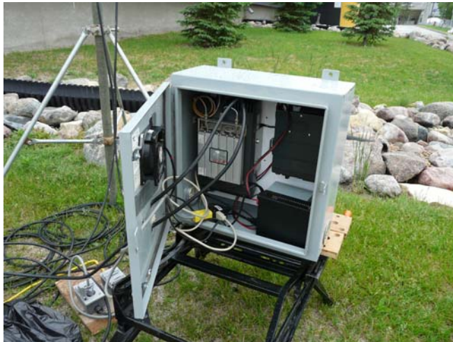
UHF Repeater Cabinet with link radio Photo Credit VE4ESX
