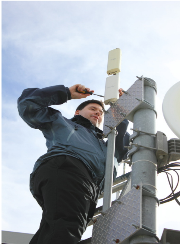
William VE4VR installing an HSMM antenna on the roof at 55 Nassau Street
