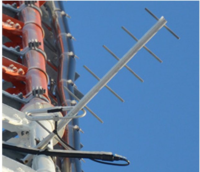
Broken antenna in need of repair
